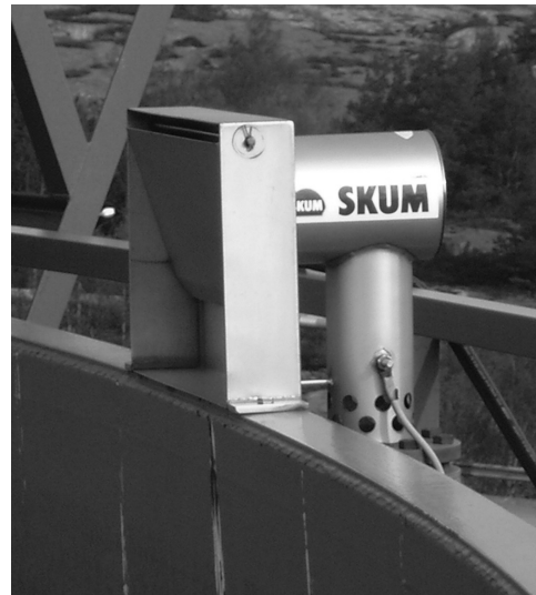
FIGURE 1 OVER-THE-TOP FOAM GENERATOR INSTALLATION
